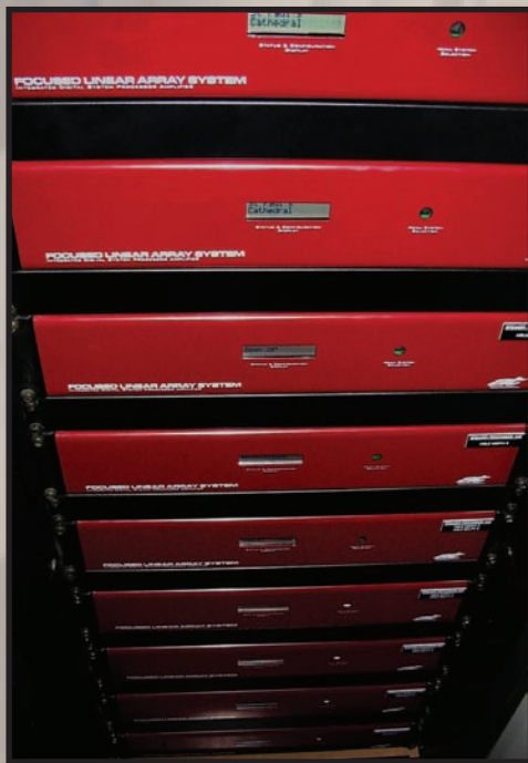
A part of the FLA8 amplifier rack in St. Paul's Cathedral
