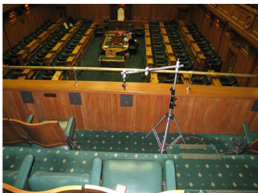
Figure 5: Balustrade Type Loudspeaker
